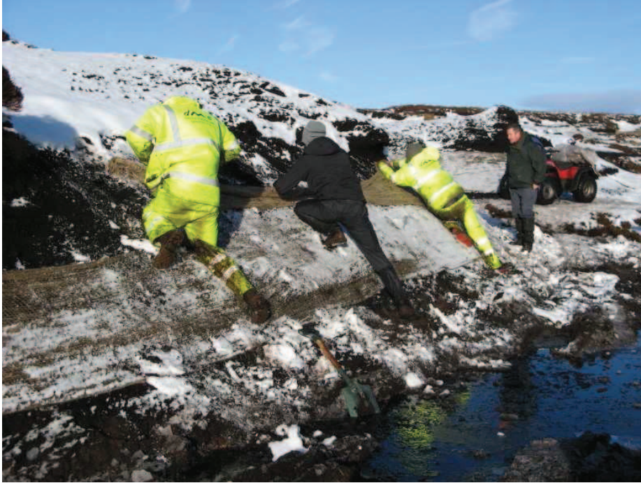
Geo-textile being installed at Langden Head on steeper slopes of bare peat to promote re-vegetation.
